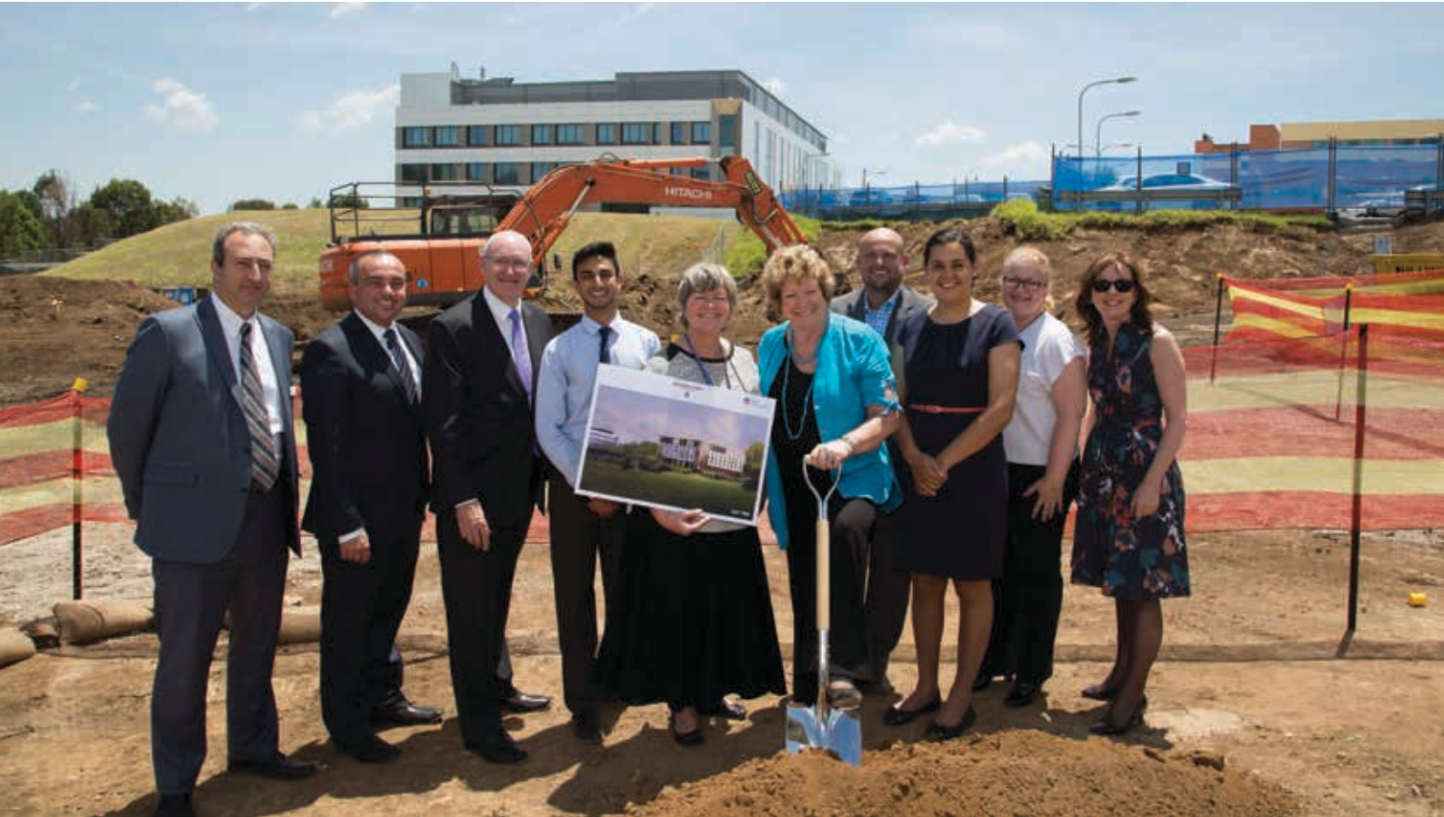
Construction begins - Construction has begun on a new clinical school in south western Sydney which will provide advanced training to young medical students and researchers. The $21 million, four-storey building is being constructed on the Campbelltown Hospital campus and is funded by the NSW Government and Western Sydney University.
