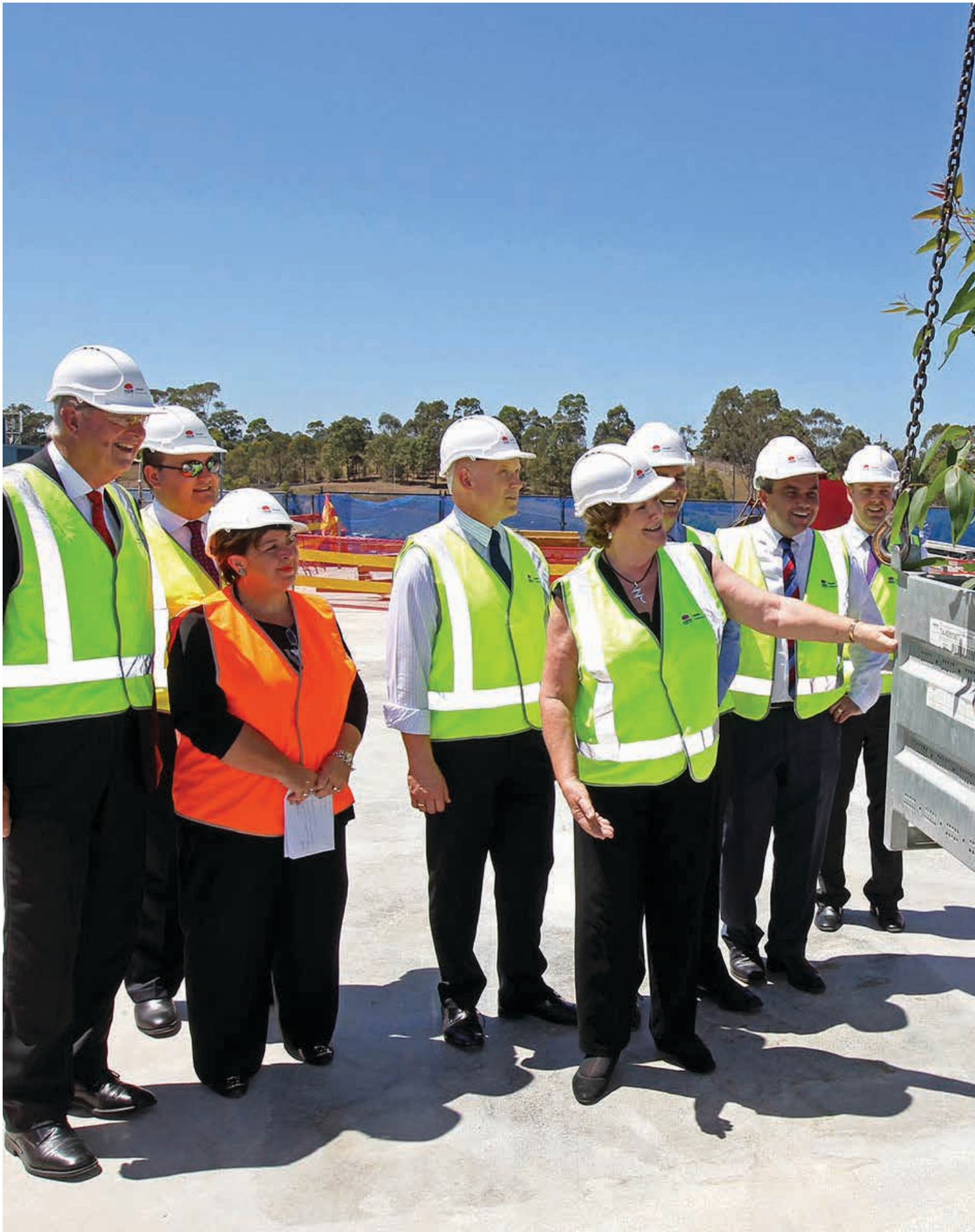
A Topping Out ceremony was held to mark completion of the highest point of Campbelltown Hospital's new multi-storey clinical services building.
